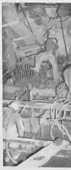
OUT OF THIS WORLD: Looking like men from out of this world, these members of the "concrete gang" of the Mechanical Department are busy putting in a new base for the No. 7 turbo-generator in the No. 1 Powerhouse. Working inches above sea-level, they're wearing fresh air masks to guard against hydrogen sulfide which seeps through the coral strata enough to discolor the eyes in their pockets. The new General Electric turbo-generator will produce 7500 kilowatts; some 200% more than the No. 5 which "went bad" in January of 1952. The new unit is expected to go into operation early next year.
